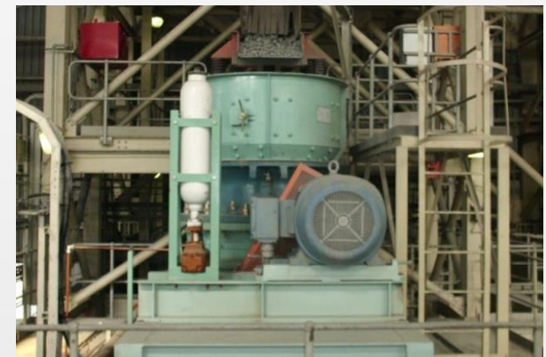
Kawasaki Cybas i1200 cone crushers installed in Letšeng's Plants 1&2
